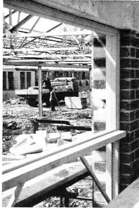
An interior view of the new Design Centre. The workmen are unloading corrugated asbestos roofing. The building will include a conference room and a library
